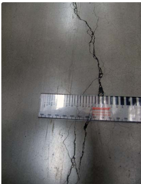
Figure 4: Damage at cracks.
