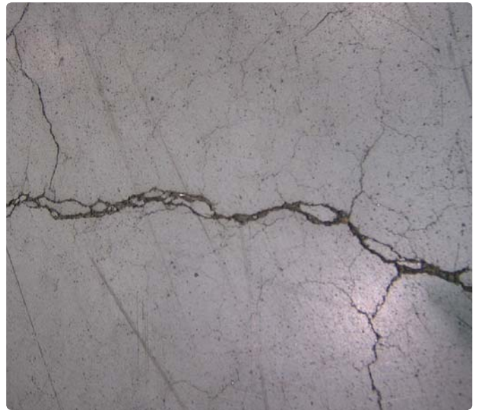
Figure 4: Breakdown of surface at cracks
